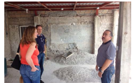
Bobby snapped a picture of my son Gary and his wife Rita (left) looking at the newly repaired wall with house parent Ramon at the boys' home in Piedras Negras.
